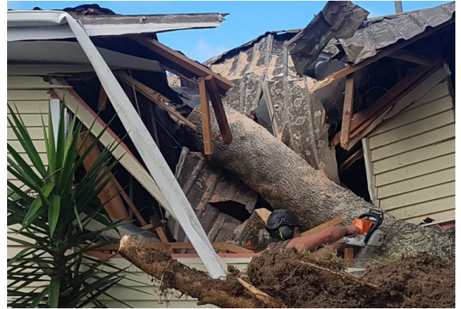
A Spencer Henshaw tradesman at work on a very large tree that caused significant damage to an Otara, South Auckland property. The damage was so extensive the tenant needed to be permanently rehoused
