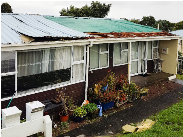
The pensioner complex in Mt Roskill where the roof was blown off
