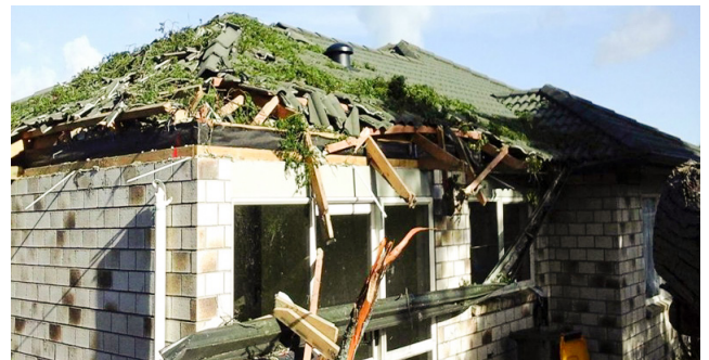
The Mangere house where the tenant’s health issues meant they were unable to leave. To allow the tenant to remain in the property and stay safe, our contractor isolated the damaged roof area by building a temporary wall inside the house and disconnected power to this part of the property. The grounds were cleared of debris so the tenant could move around safely. This effort was another example of the lengths our contractors went to during this storm and its aftermath.
